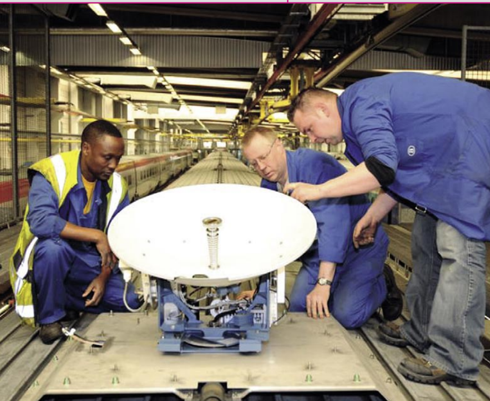
21net technicians at work installing the SeaTel satellite antenna for the mobile reception of HISPASAT. Since the Thalys high-speed trains don't travel much up or down any hills, the antenna itself doesn't require much in the way of elevation adjustments. This results in a lower wind load thanks to the flatter radom.
