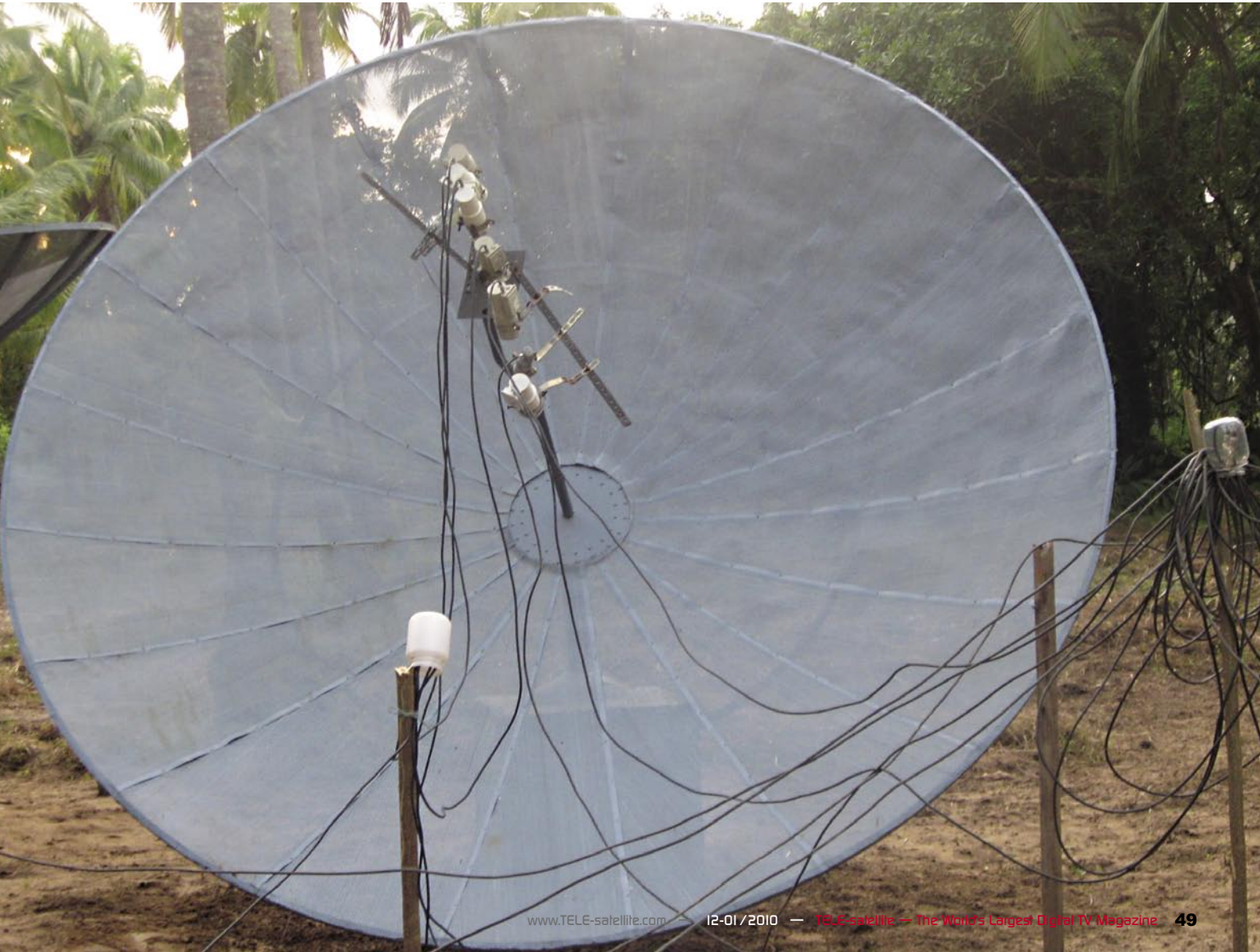
■ All is cleared and the LNBS are ready again for connecting to the receivers.
